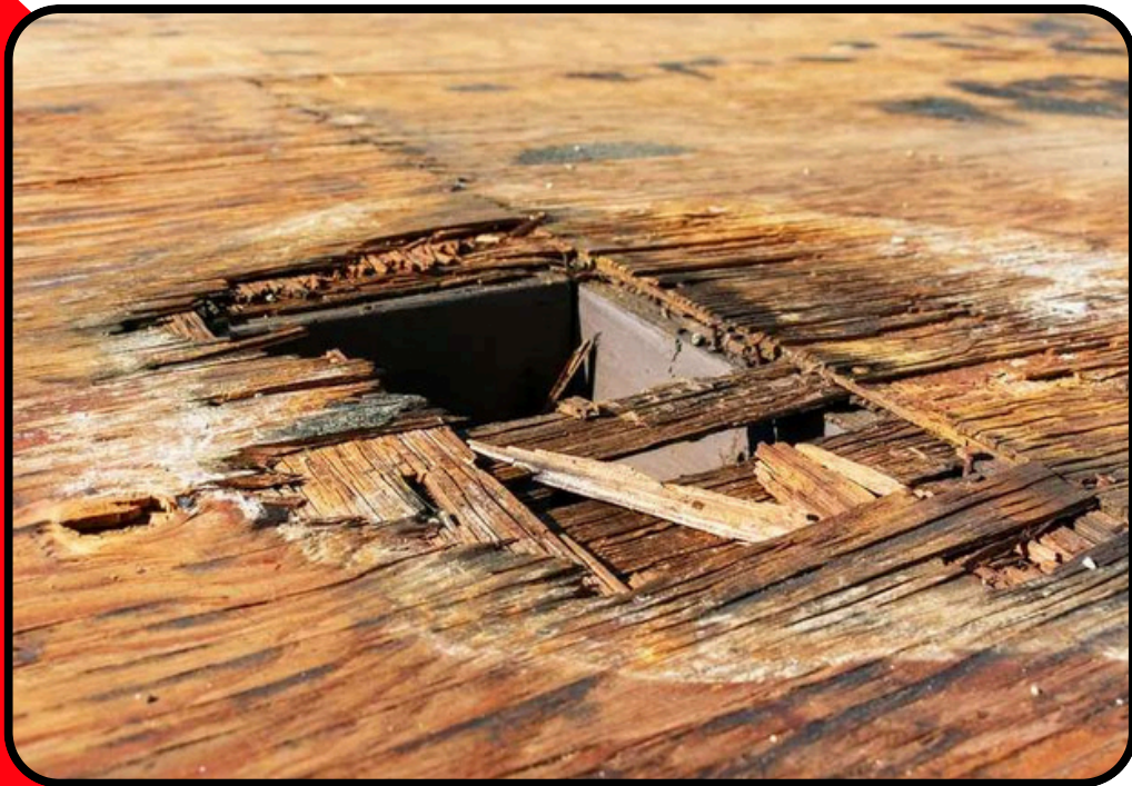
↑ EXAMPLE OF DAMAGED ROOF DECK
