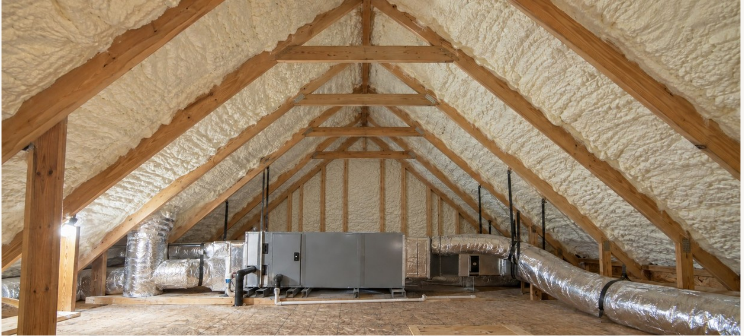
Attic HVAC equipment
